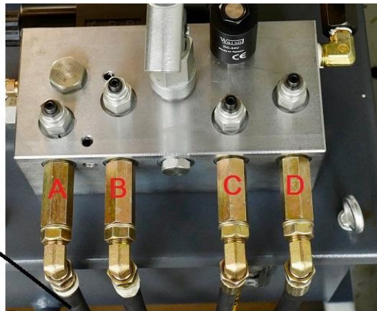
Connection of hydraulic hoses inside of the cabinet
